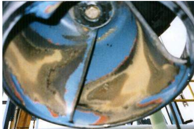
Erosion on suction side
