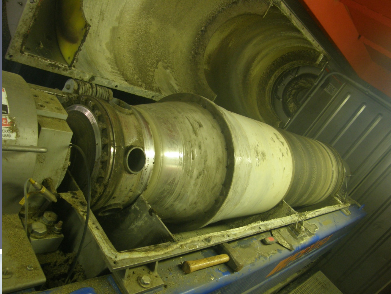
Centrifuge - Dane County Digester; Clear Horizons
