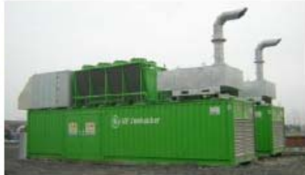
2 x containerized J420 fueled with coalmine gas at Huainan, China
