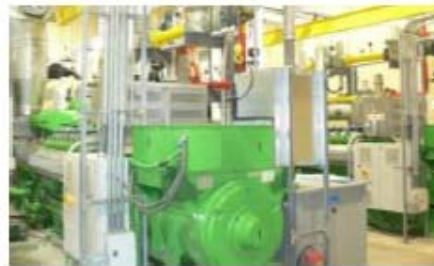
2 x J420 fueled with sewage gas at Bergen WWTP, USA
