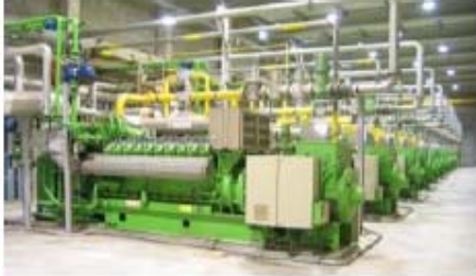
11 x J420 fueled with landfill gas at Pinto, Spain
