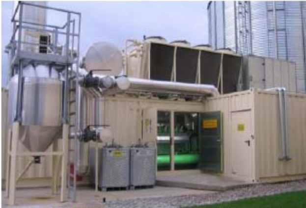
Picture: Example Type 4 biogas container
