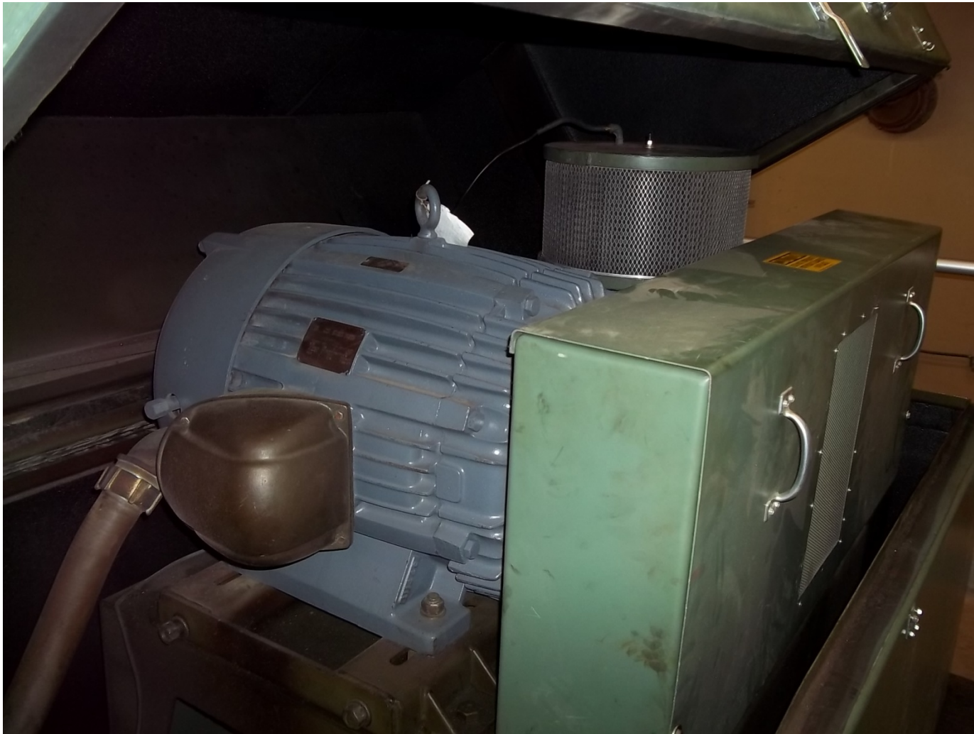
75 hp motor installed
