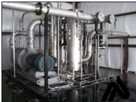
1,600 scfm Biogas Conditioning System for CAT engines
