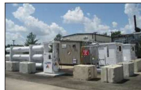
Upgrade to a BioCNG™ 50 Permanent Storage and Fueling Station
