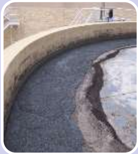
Create Gas (Primary Digester)
