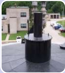
Store Gas (Secondary Digester)
