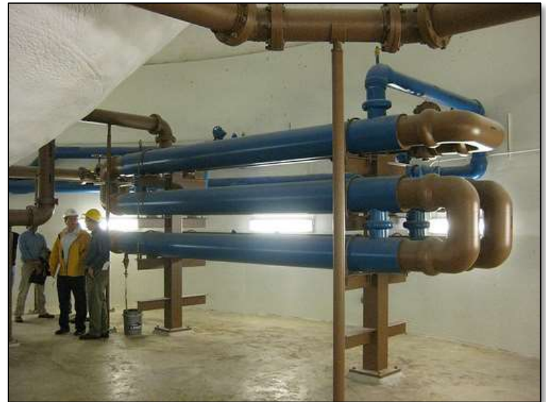
CB&I-Supplied Tube Heat Exchanger
