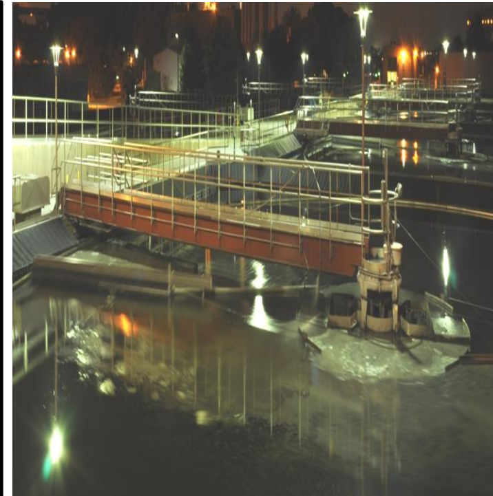
NEW Water Wastewater Treatment Facility
