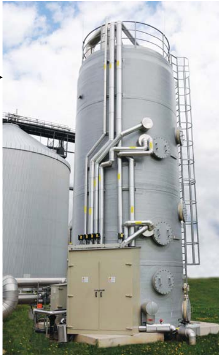
Biological Scrubber Hydrogen Sulfide Removal
