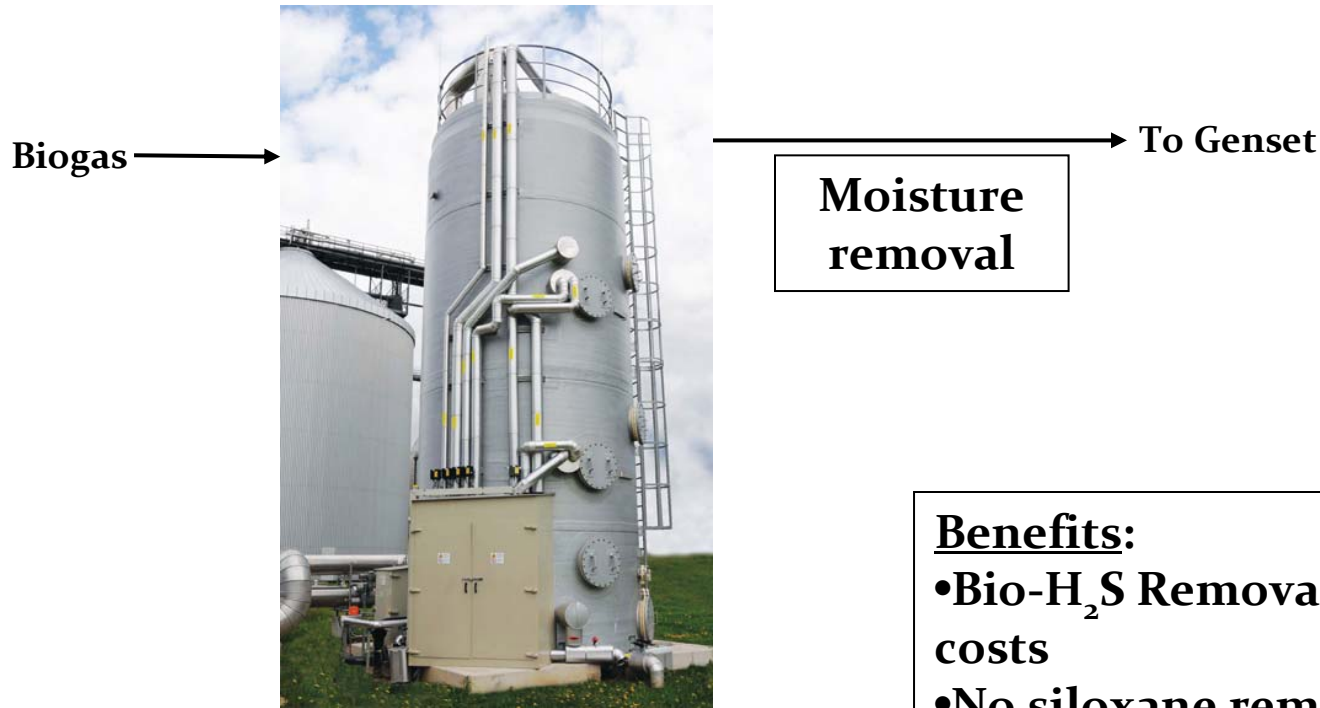
Biological Scrubber Hydrogen Sulfide Removal
