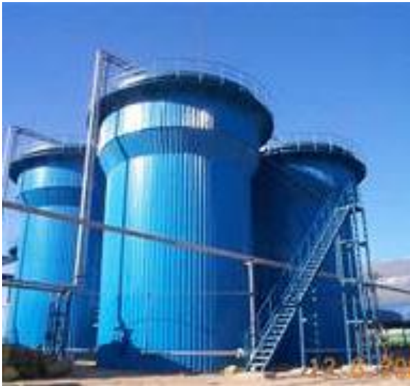
Industrial Waste Digester
