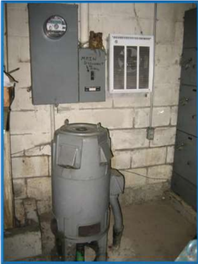
Deficient Pumps & Controls
