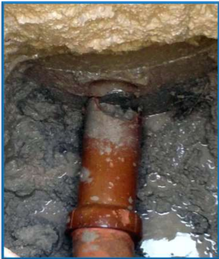
Hole in pipe near manhole connection
