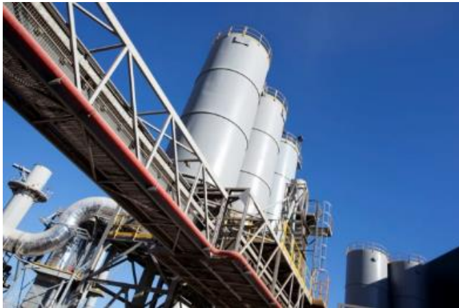
Dried sludge silos and transport to cement kiln
