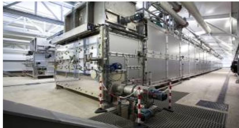
View of the drying tunnel inside the building
