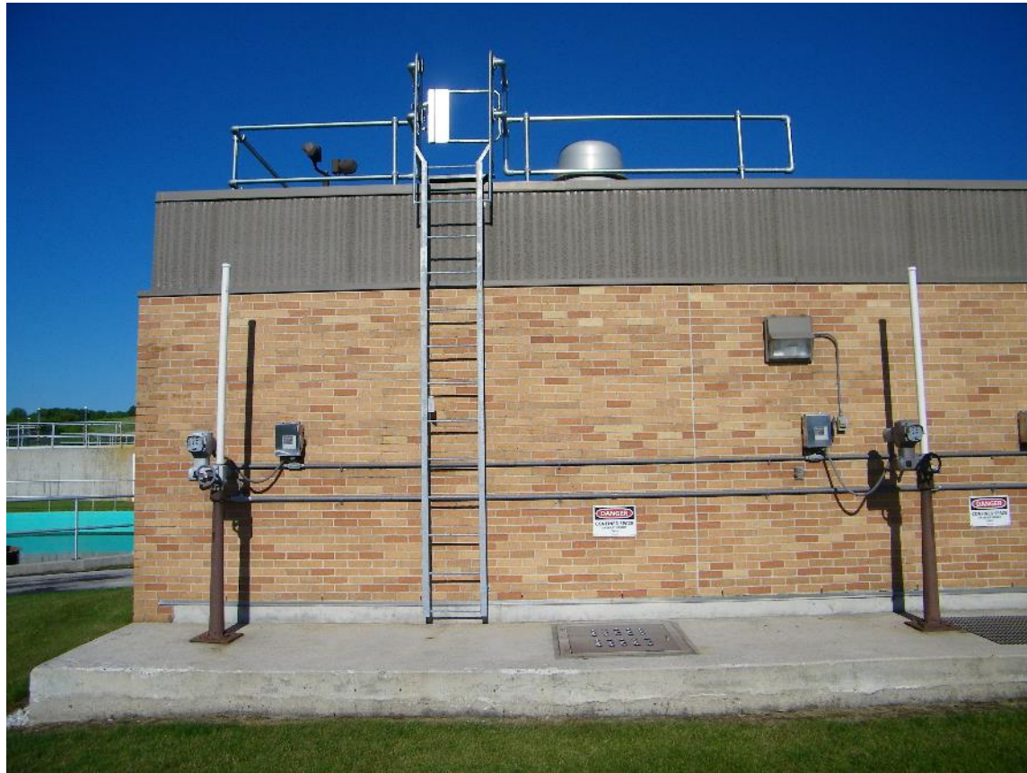
Fixed Ladder with Railing
