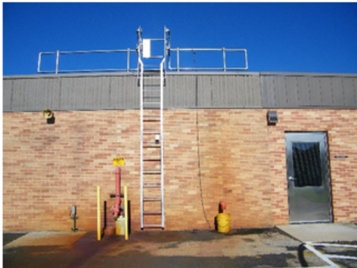
Fixed Ladder with Guardrail
