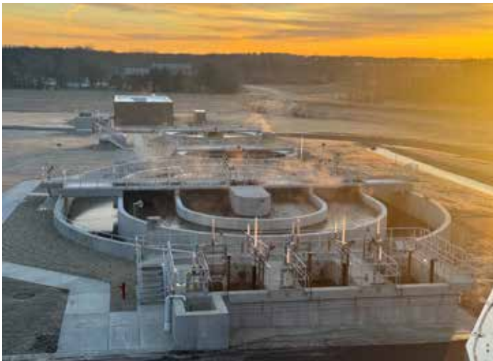
Figure 6 Sunrise over the Ixonia oxidaton ditch
