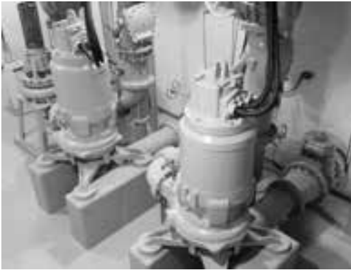
Newly installed pumps
