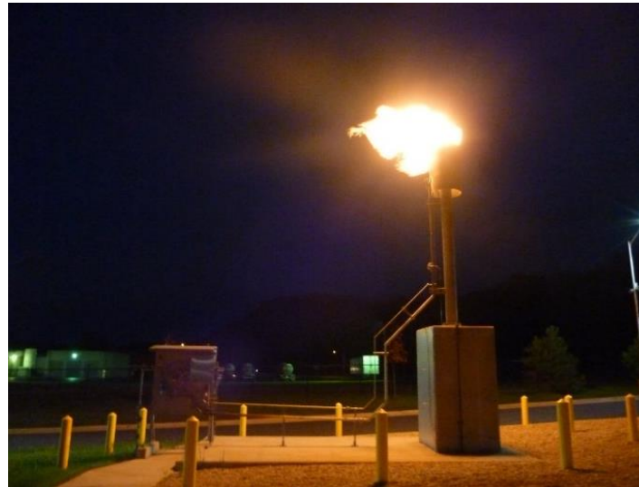
Waste Gas Burner
