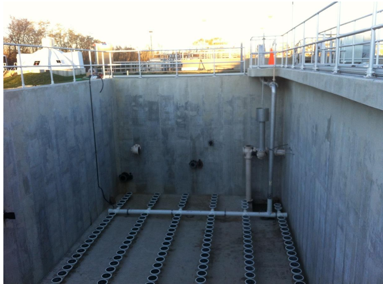
Lake Barrington IL, Aerobic Digester
