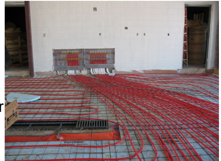
Infloor radiant heat
